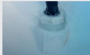
Cable gland not sealed
