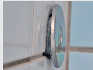
Nozzle is at an angle in the pool wall
