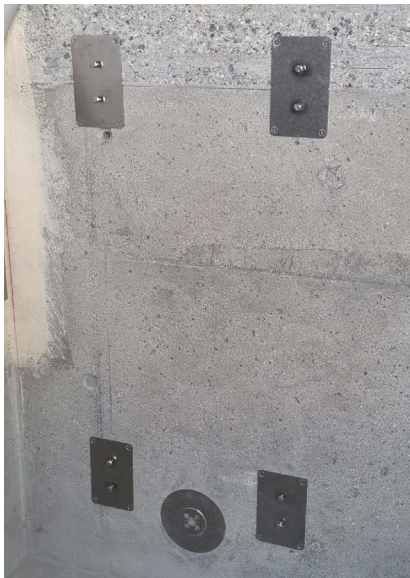
7. Mounting flanges for a ladder
