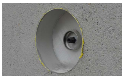
6. Screwed out: It has no rusty nails
